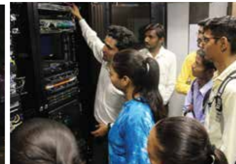
BSNL Ahmedabad Networking & Telecommunication server room
