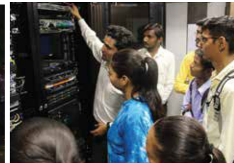
BSNL Ahmedabad Networking & Telecommunication server room
